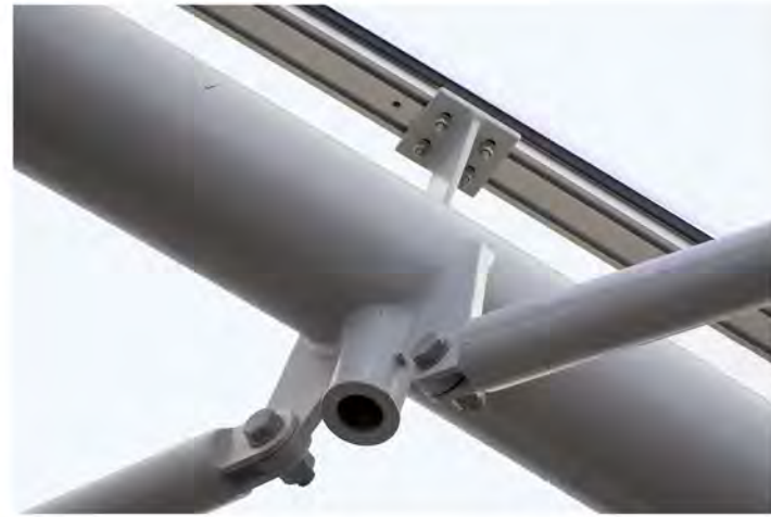
Bottom A cross-section of the 6-inch extrusions mounted on the steel arches of the lattice shell structure. A round channel and clamp bar hold the edge of the ETFE foil in place.
