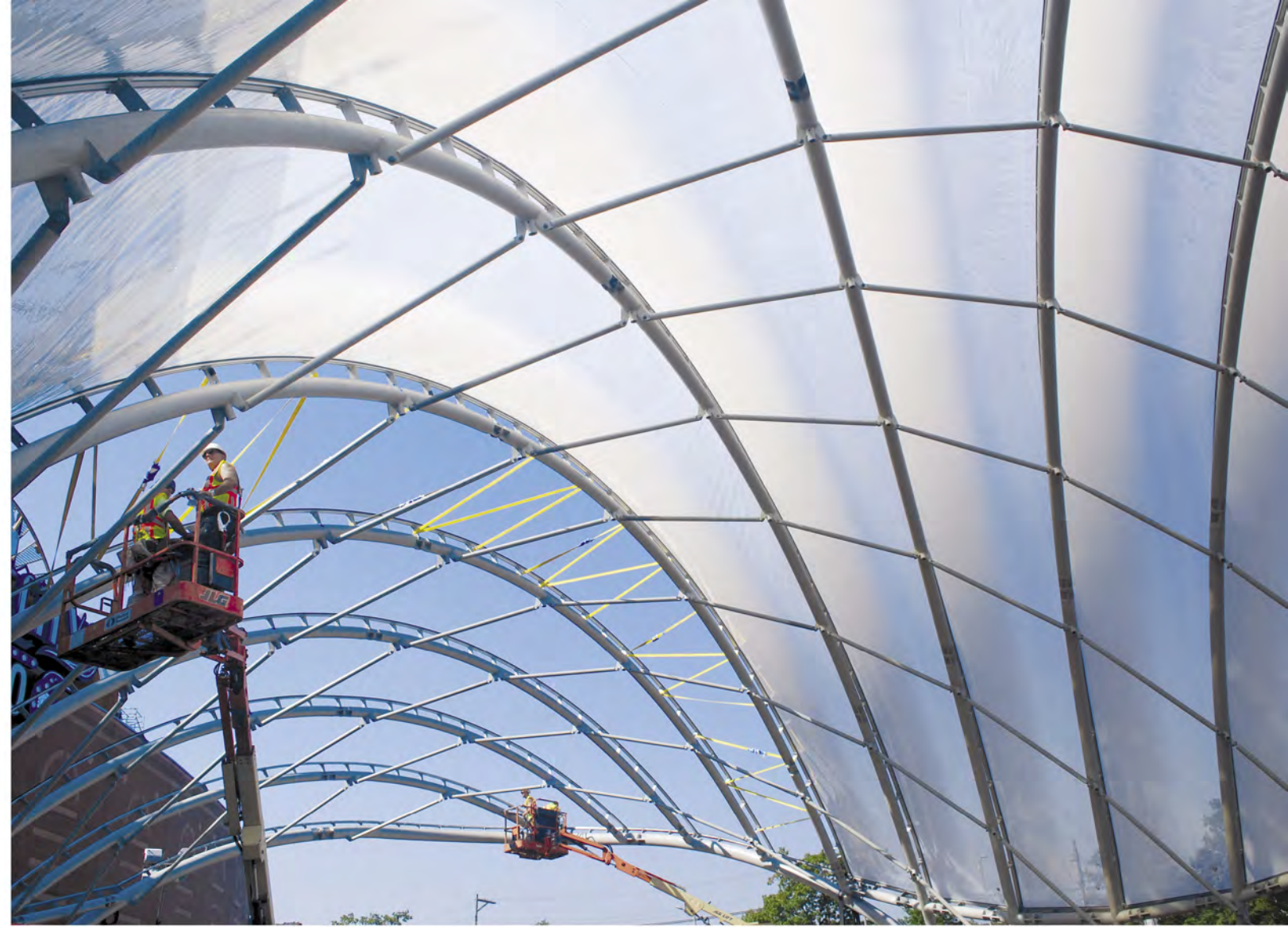
This spread The 11,000-square-foot porte-cochère is a steel lattice shell structure covered with ETFE, a transparent film that is lightweight, flexible, and sustainable. Installers feed the edge of the ETFE film into the clamp bar of a 6-inch steel extrusion designed to hold the material in place.
