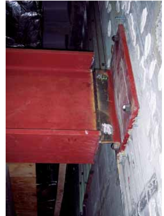
Top On the north side, the beams attach to a 36x8x1.25 HSS that transfers loads to the building's columns. Bottom On the south side, the beams attach to imbeds in a shear wall.
