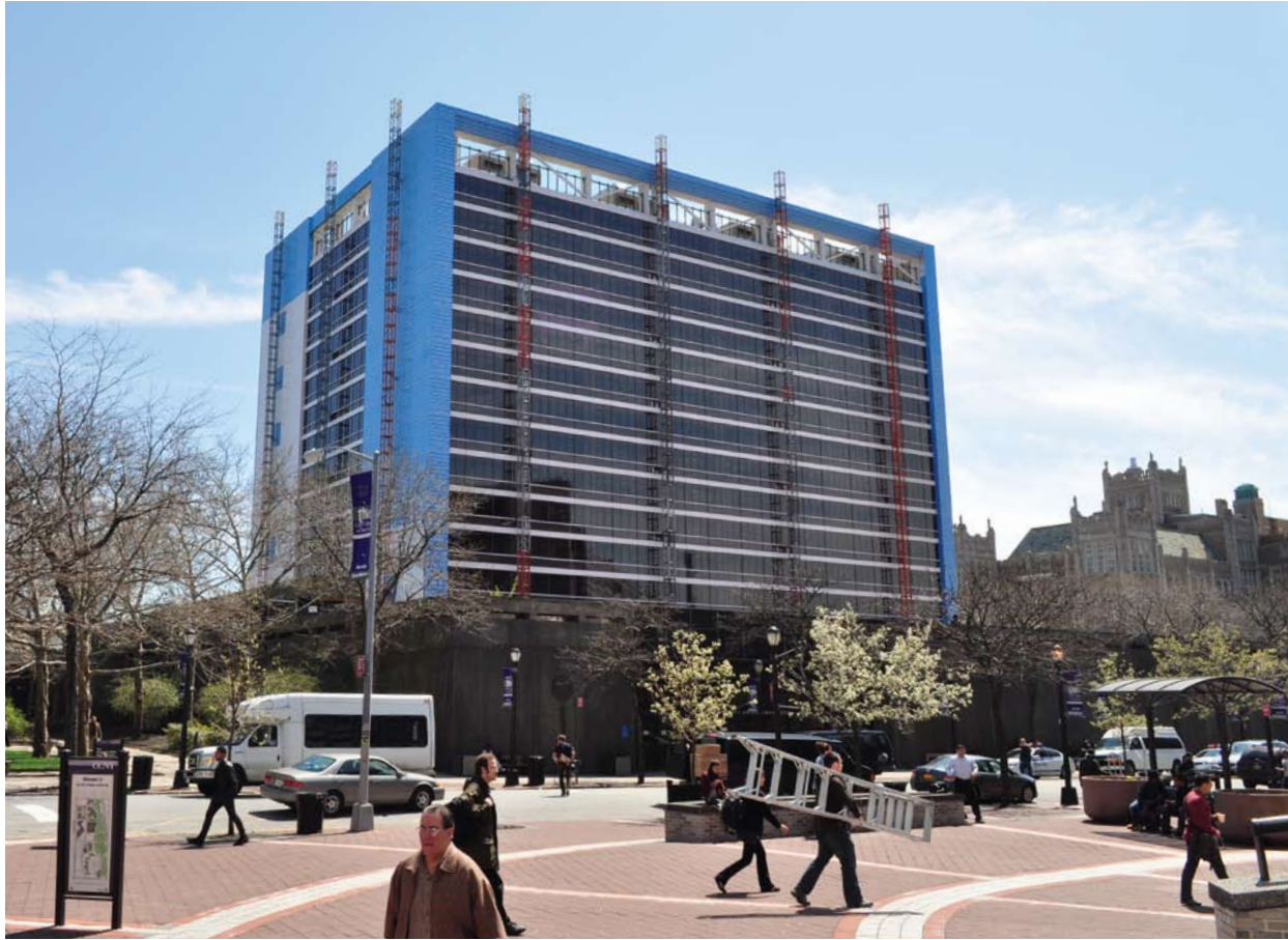
Above Recladding the Marshak building will increase its energy efficiency and prevent further deterioration of its 40-year-old lightweight concrete facade.
