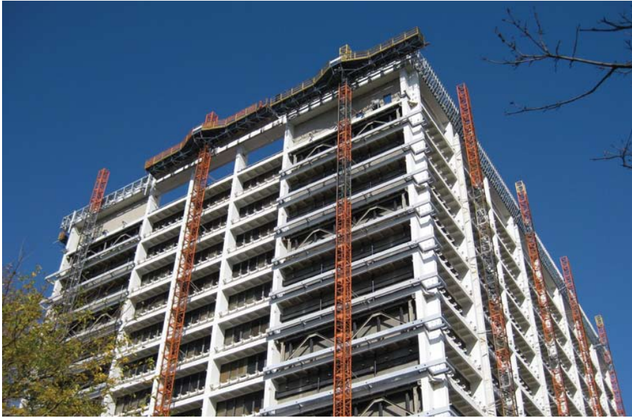
Above HSS box sections spanning between columns will transfer the curtain wall load directly to the existing columns without transferring any new load to the slab edges.
