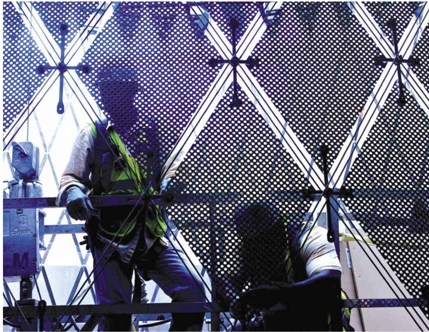
Above Three teams of contractors performed the panel installation, connecting each panel to nearby cruciform at its four corners.
